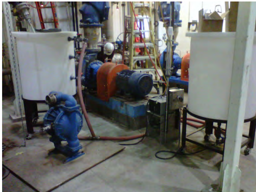
Figure 6: High Salt EQ Tank pilot plant. One 100 gallon reactor.
