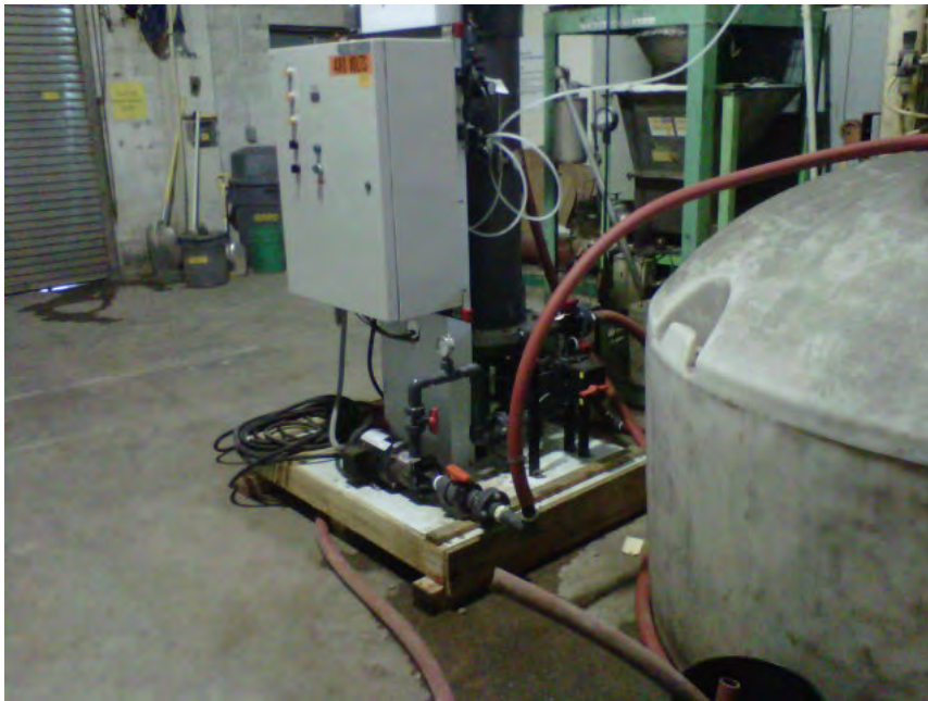
Figure 19: Kroff One pass MF at ADM Pilot plant
